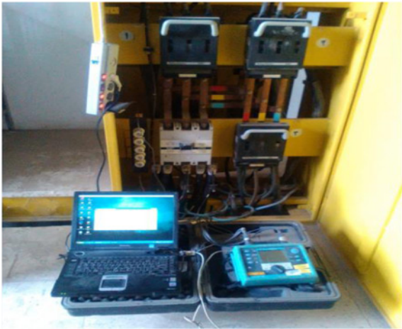
Fig. 3 Power analyser which is used in Golestan complex substation
