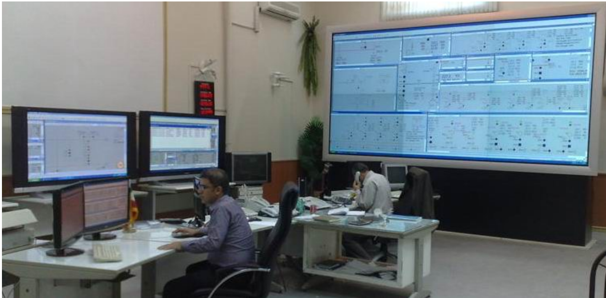
A regional SCADA, West Regional Electric Co., Kermanshah (Aug. 2009)
